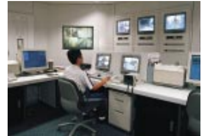
Central Monitoring Stations
