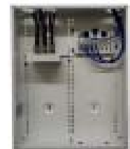
Structured Wiring Cabinet
