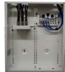
Structured Wiring Panel
