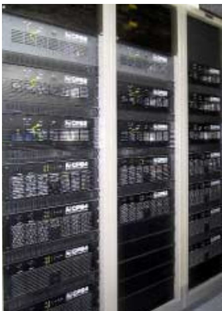
Concentration of power: the CPS amp racks.
