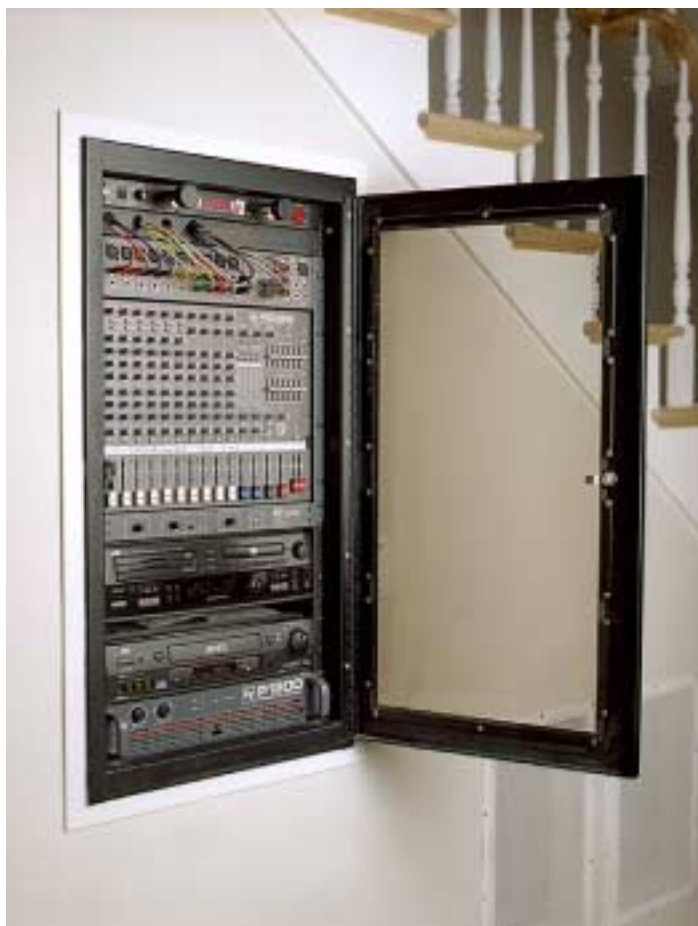
The main control rack houses the PSX1000 powered mixer, the XP200a low-frequency processor, and the P1200 amp.
