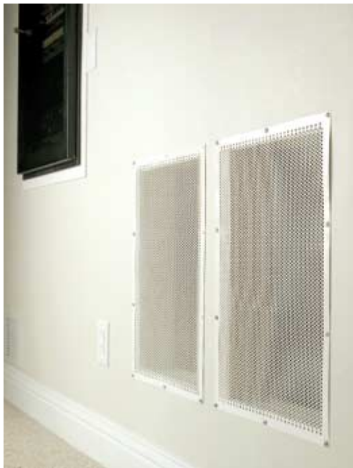
Two Sb subs are built in under the staircase by the main control rack.
