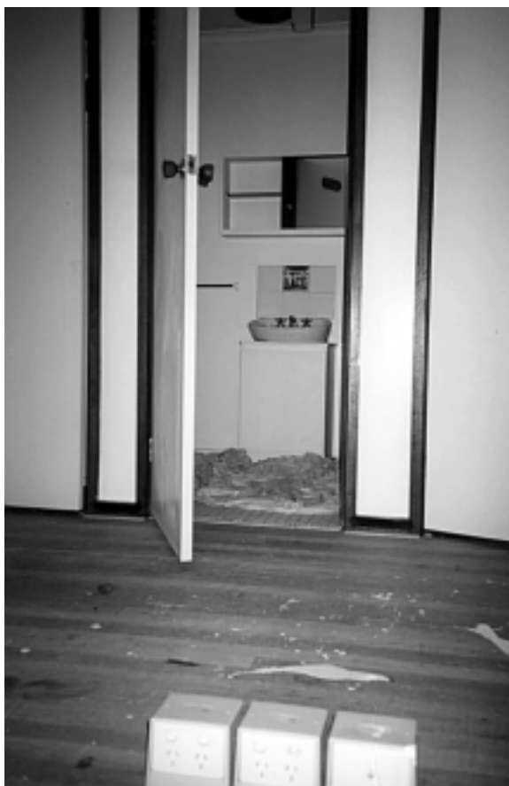
House in progress. Elaine's new study before the carpet went in, and before some repairs to the en suite (through door). The three boxes are the new telephone connection and power points. (Photo: Yvonne Rousseau, 23 September 2004.)
